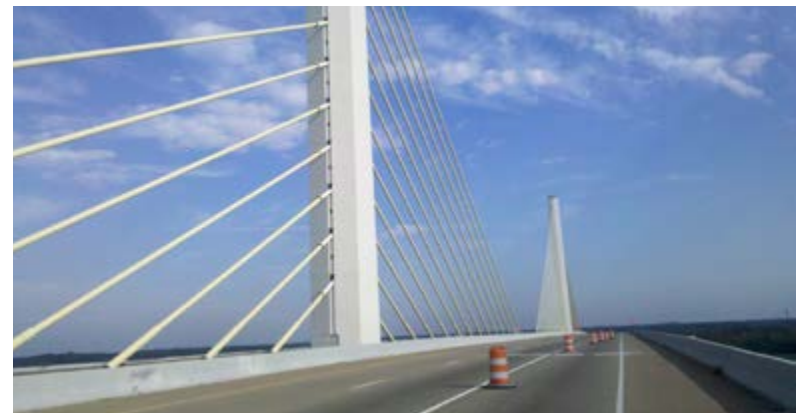
Varina-Enon Bridge under construction. Left and top photos courtesy of VDOT. Bottom photo courtesy of Nico DeLeon.
